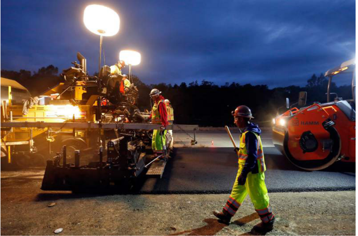
The DeSilva Gates Construction crew on an immense asphalt paver, left, applies base layers of material on the number one lane of southbound Highway 101 as a vibration roller and other support personnel follow behind, near Geyserville, California, on Wednesday, May 16, 2018. (Alvin Jornada / The Press Democrat)
